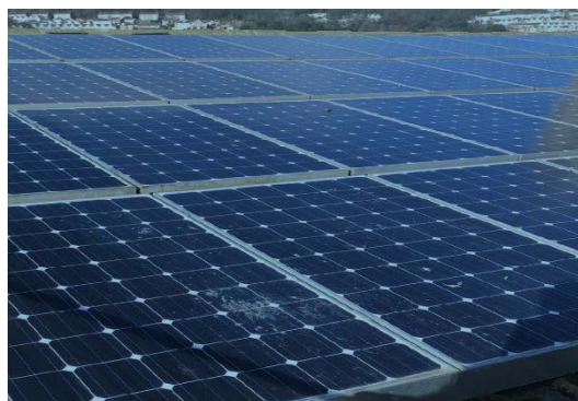
Solar PV modules installed on the Guildhall
